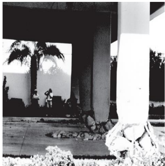
Figure 2: Crushed columns at base of Imperial Country Services Building (U.S. Geologic Survey)
